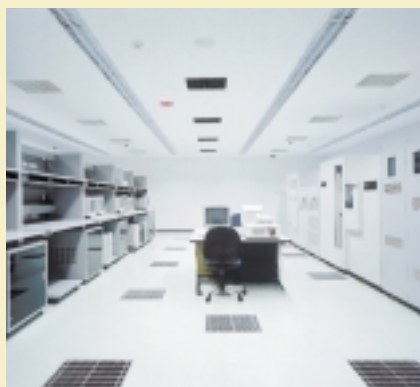
Information Center Computer Room
