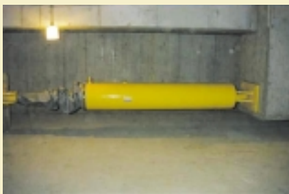
An oil damper of the base isolation system, which is placed in the base. The damper's right-hand end is fixed to the building's main structure, and the left-hand end is fixed to an anchor block on the base.
