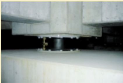
The base isolation system in completion
