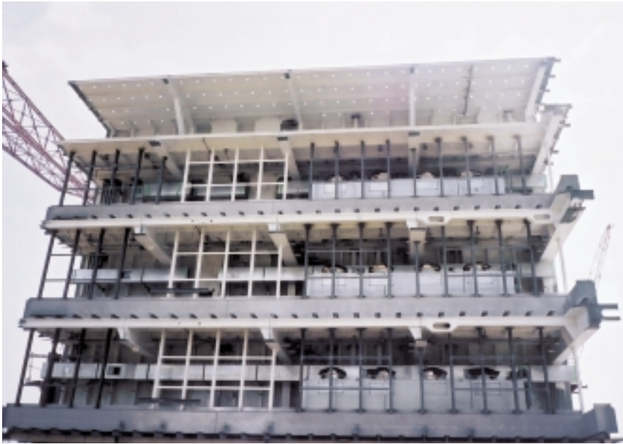
Refrigeration units built into a section of the PCC
