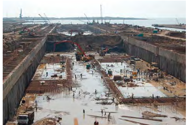
When completed, Pipavav Shipyard's drydock will be the largest on the subcontinent.
