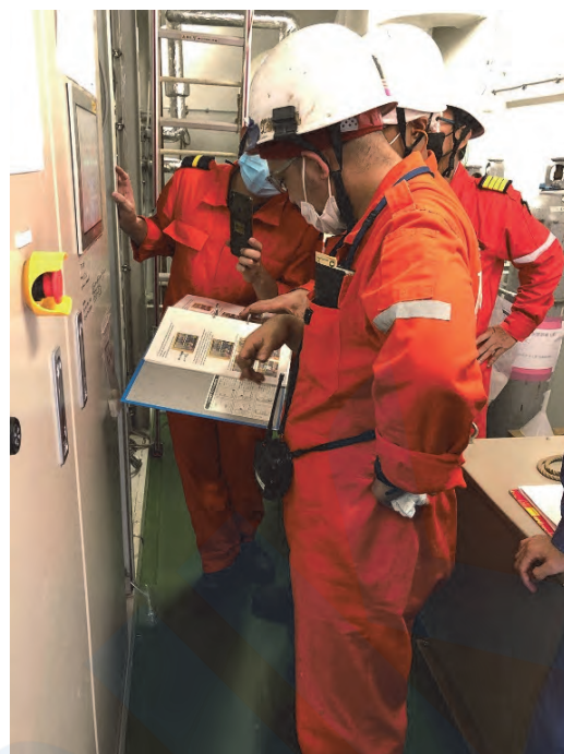
Fig. 10 Operation of demo plant by ship's crew
