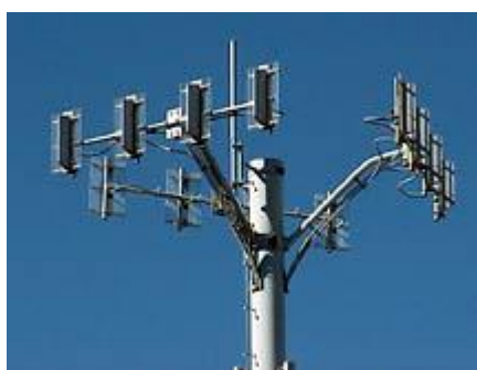
Figure 1: A mobile telecommunications mast with three aerials – therefore three "sectors"
