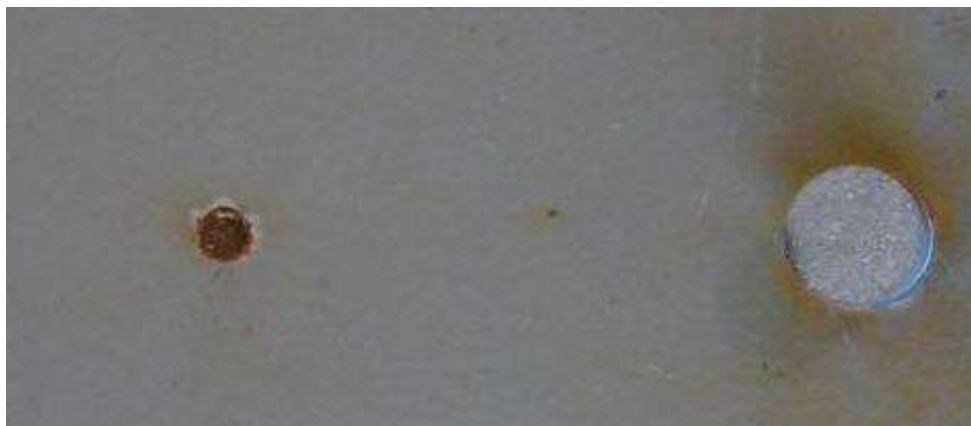
Figure C-2 Disbonding from artificial holiday, bottom wave tank panel (example picture not connected to example results in this model report).
