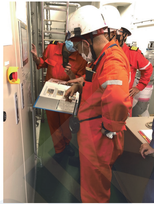
Fig. 10 Operation of demo plant by ship's crew
