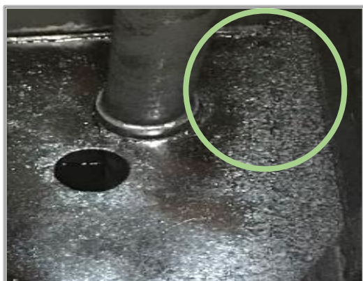
Sedimentary oil sludge at the edge of tank / between the floor space and wall surface.
