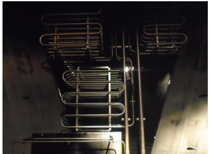
4. Heating coils close-up
