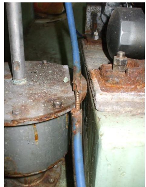
손상된 Release cable
