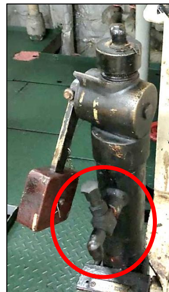
Example of small-diameter self-closing control cock
