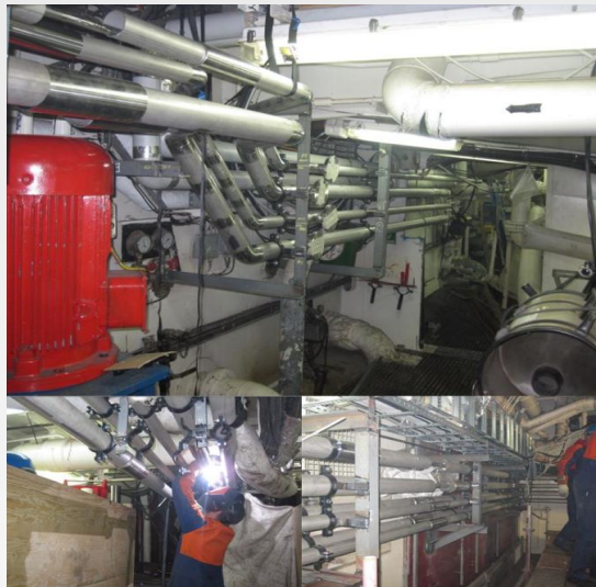
High pressure pipes
