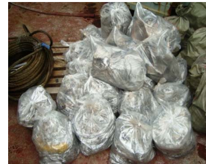
Asbestos packed in double bags
