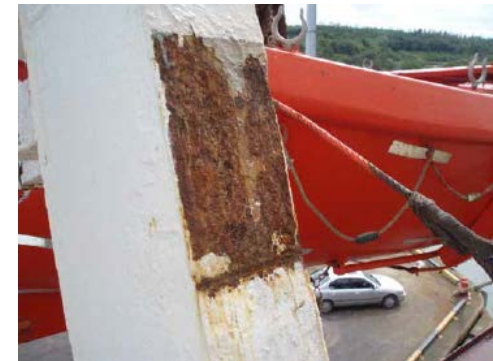
Corrosion of davit
