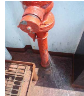
Leakage of fire line
