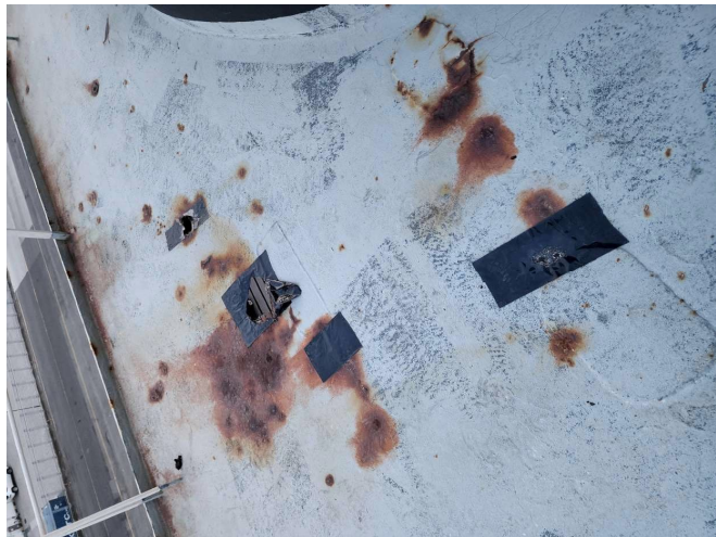
Corrosion of exposed deck with hole formation
