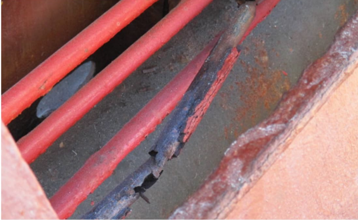
Corrosion and damage of CO 2 fire extinguishing line
