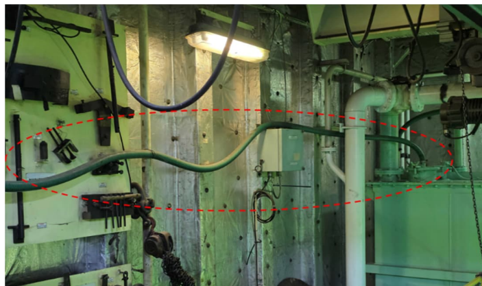
Improper piping connection to sewage treatment unit (Improper Modification)
