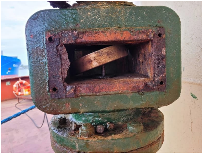
Corroded air pipe
