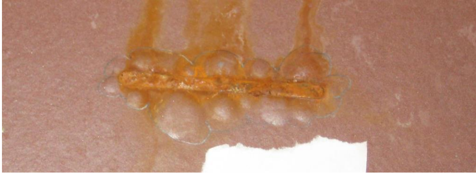
Figure C-3 Scribe area of top wave tank panel before removing of loose coating (example picture not connected to example results in this model report).
