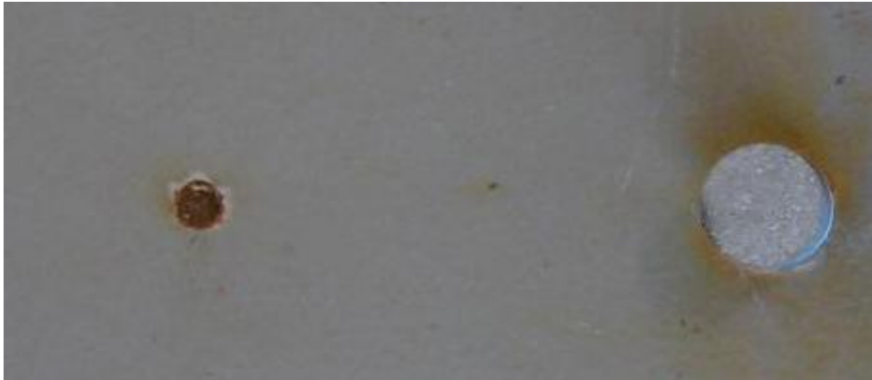
Figure C-2 Disbonding from artificial holiday, bottom wave tank panel (example picture not connected to example results in this model report).
