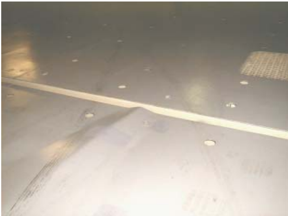
Photo 2. Abnormal deformation of Deck Plate (凸)
