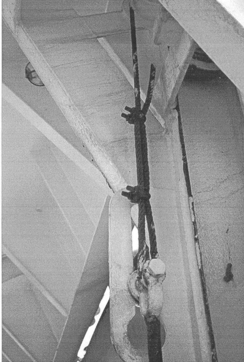
Termination is by cable grips without a ferrule and the end of the wire rope is unsecured.
